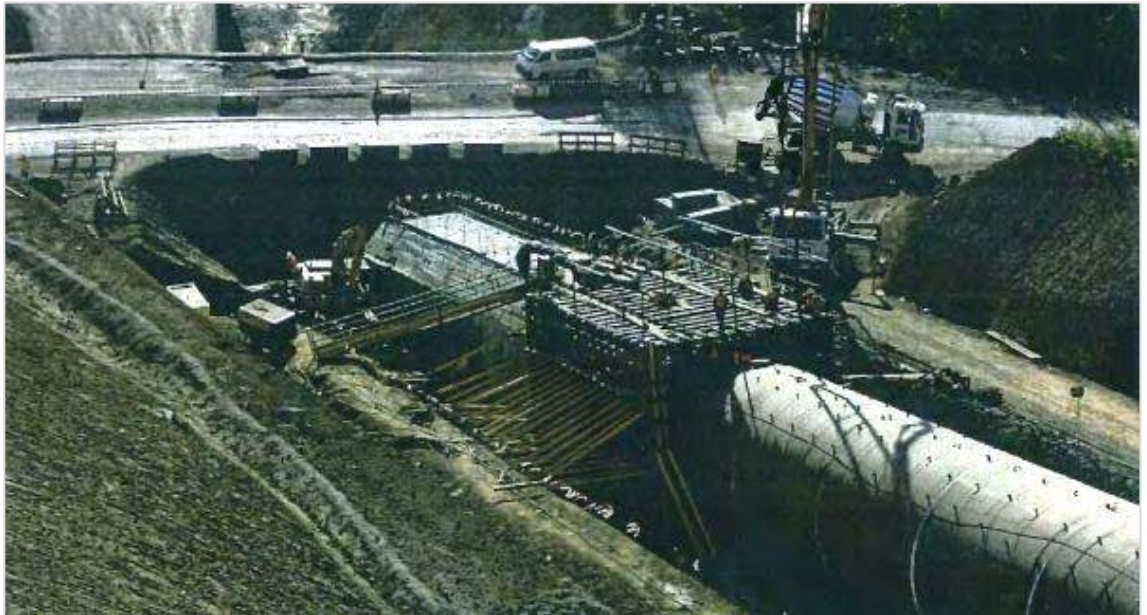
Figure 46 - Illustration of penstock construction stages - Taken from another project. Top right: concrete slab in bottom trench, Top left: installation of the penstock steel liners Bottom: reinforced concrete box over the penstock steel liners Source: Salini Impregilo
